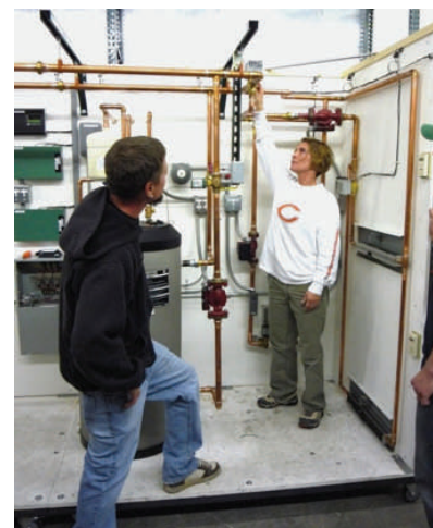
Spokane Apprentices Terry Douglas & Trish Matthews watch a proportioning valve modulate during systems training.
